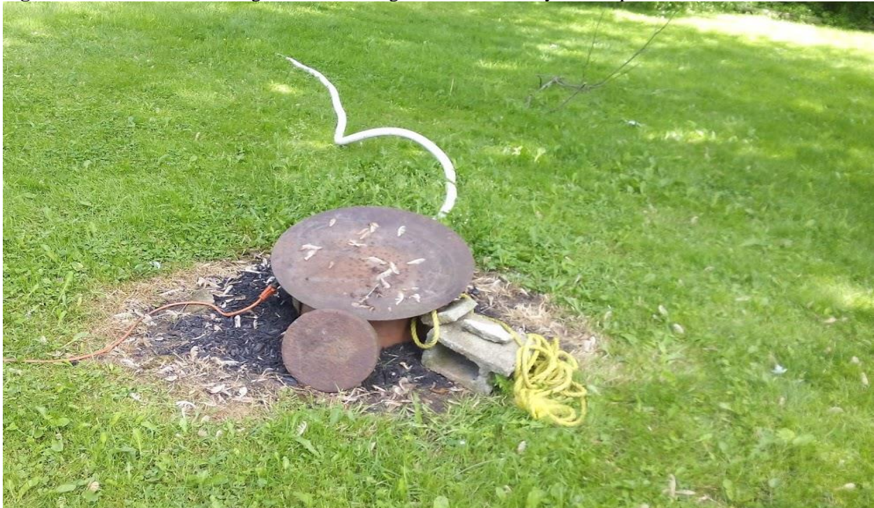
Figure 13: HSTS Illicit Discharge Detected during Class I Aeration System Inspection
